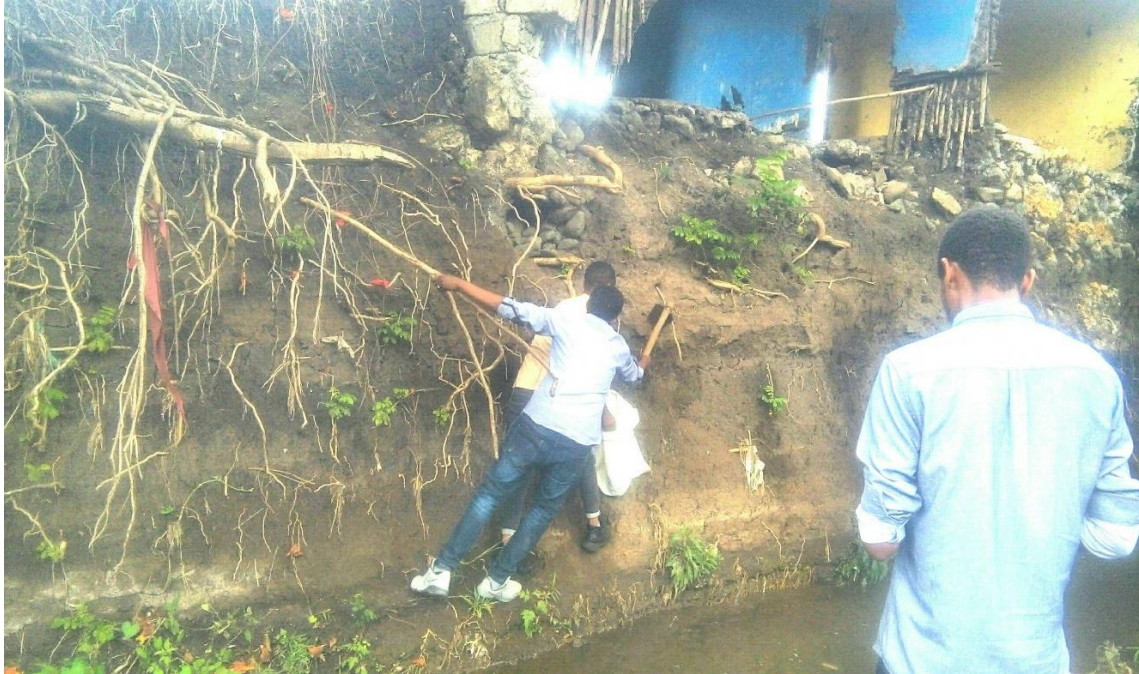
Figure 16. Unconsolidated and non-cohesive bank materials at the lower reach.
